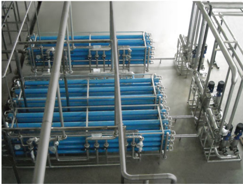
Figure 9. Reverse osmosis plant in Thailand, 230 \text{ m}^3 \text{ h}^{-1} (by EUWA).
