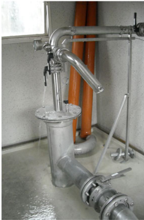
Figure 1. Wellhead of an underground water source in Central Europe, 120 m depth, capacity approximately 15 \text{ m}^3 \text{ h}^{-1} (by EUWA).
