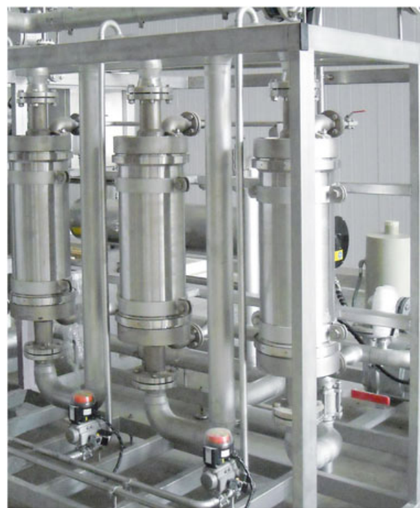
Figure 12. Membrane-based deaeration system in Thailand, 50 m 3 h -1 (by EUWA).
